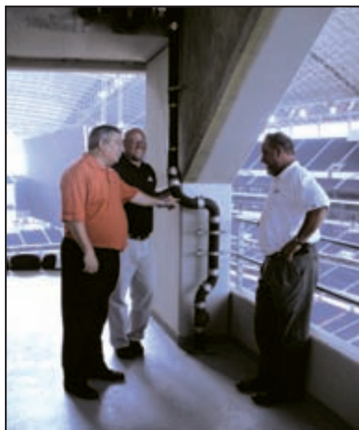
Tyler Pipe’s Bill Bliss, Sterling Bowman and Bob Davis point out some of their cast iron pipe used in construction of the new Cowboys Stadium. In all, Tyler supplied close to 5,000 tons of pipe.
