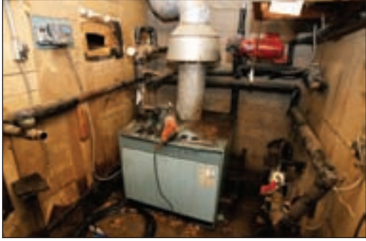
The complex's 6'x10' boiler space presented a challenge to Advanced technicians, who turned this shambles into a neat, organized mechanical room.
