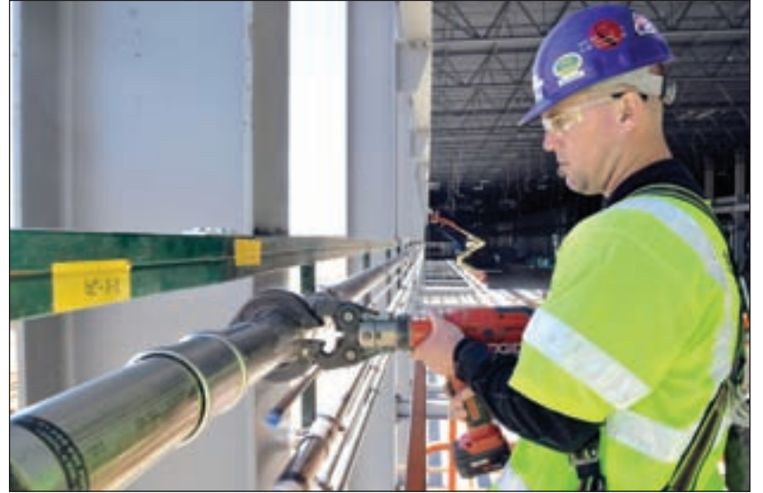
Fifty Olson employees piped the Vestas facility in just five months using the Viega ProPress Stainless System.
