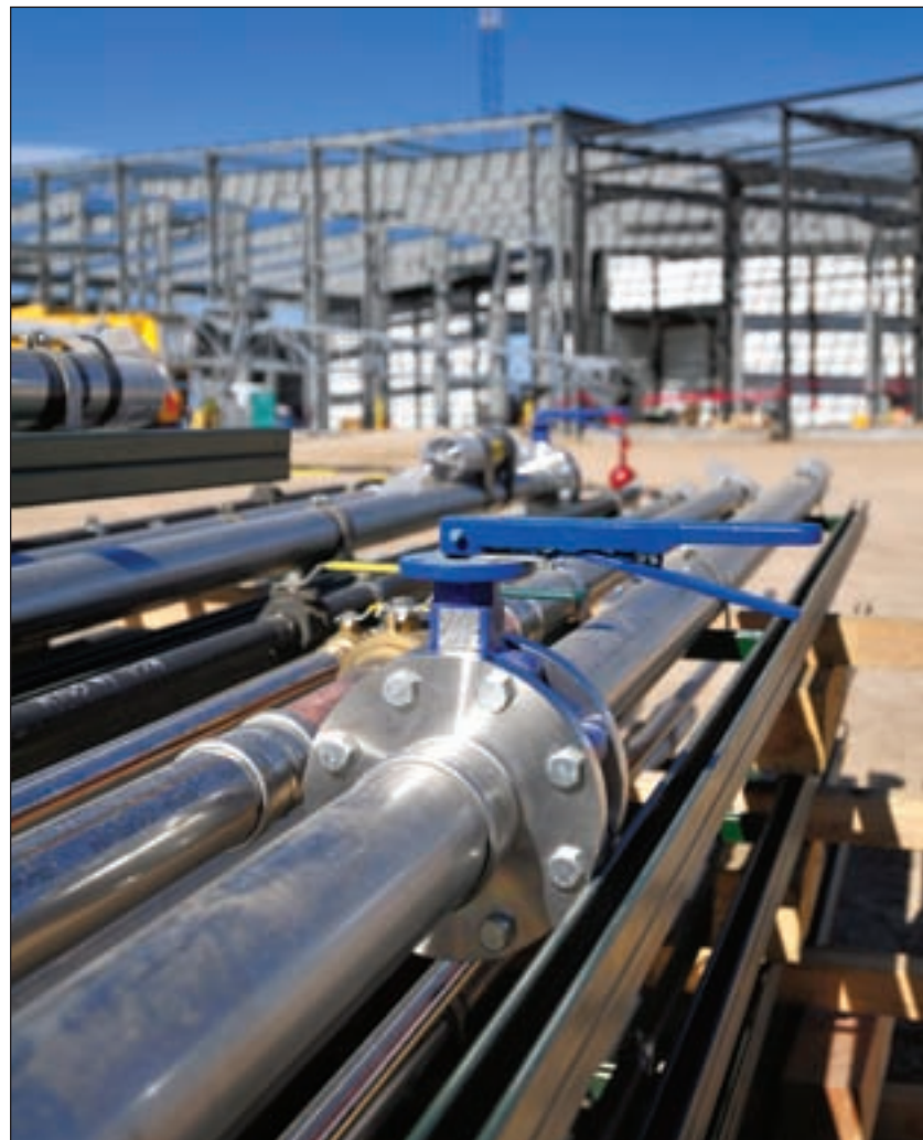
Olson Plumbing & Heating uses the Viega ProPress Stainless System exclusively, as shown in this prefabricated industrial gas and compressed-air piping section waiting for installation at the Vestas wind-tower manufacturing facility.
