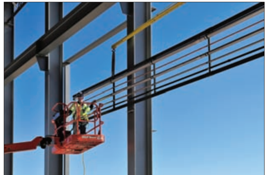
Olson prefabbed piping sections in 40-foot lengths and installed them at the Vestas facility using the Viega ProPress Stainless System.
