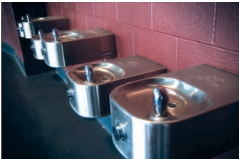
In all, Elkay custom-designed 149 sinks, water coolers and fountains with the "M" logo and completed the project in 40 days.
