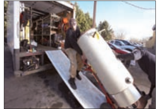
Advanced techs load up an old, leaking water heater, to be replaced by a 120-gallon Bradford White indirect water heater coil.
