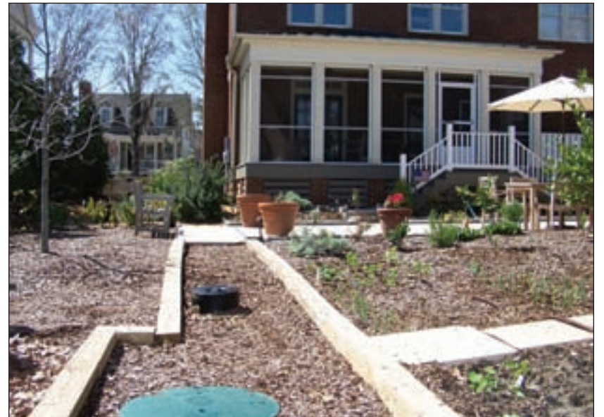
The rainwater harvesting installation is unobtrusive, with only the top of the vortex filter left deliberately visible because it helps educate visitors on how practical and important it is to re-use rainwater.
