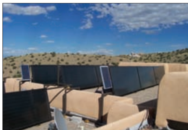
Figure 16-1. Rooftop collectors of a combi-system.
