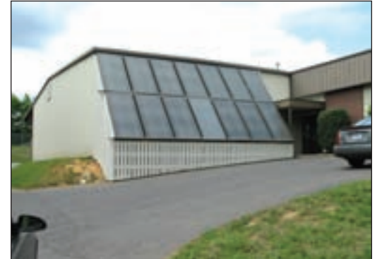
Beavers Brothers' shop sports a 14-flat-panel collector array installed 20 years ago that supplies most of the energy for radiant slab heat.
