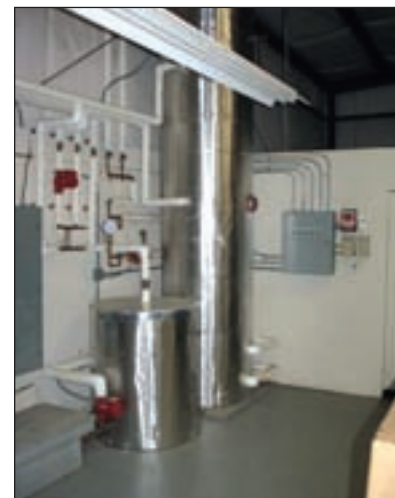
A tall, narrow, custom-built, 300-gallon pressurized drainback tank takes advantage of stratification.
