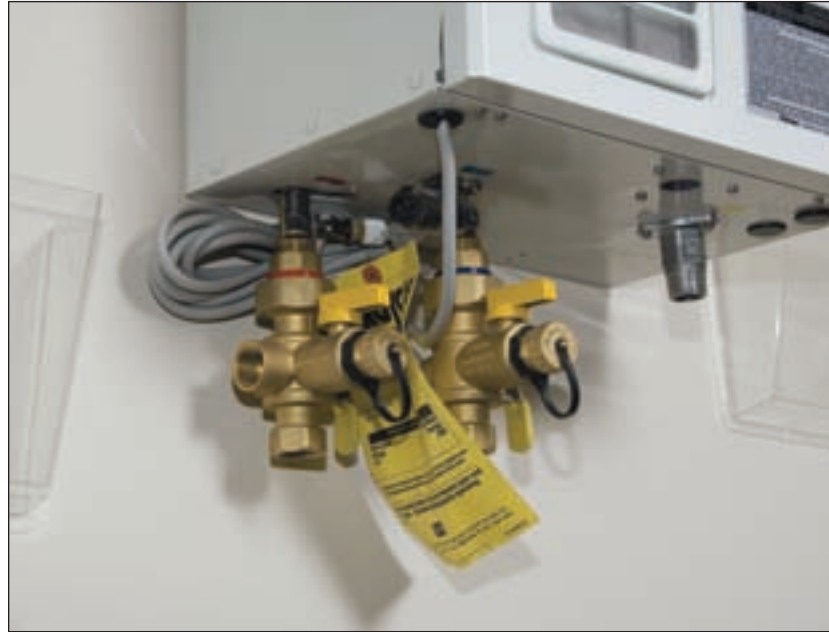
Isolation valves such as these are used by Cook Plumbing to service tankless units, such as for flushing the system of lime deposits. The frequency of this procedure depends on the hardness of the water in a locale.
