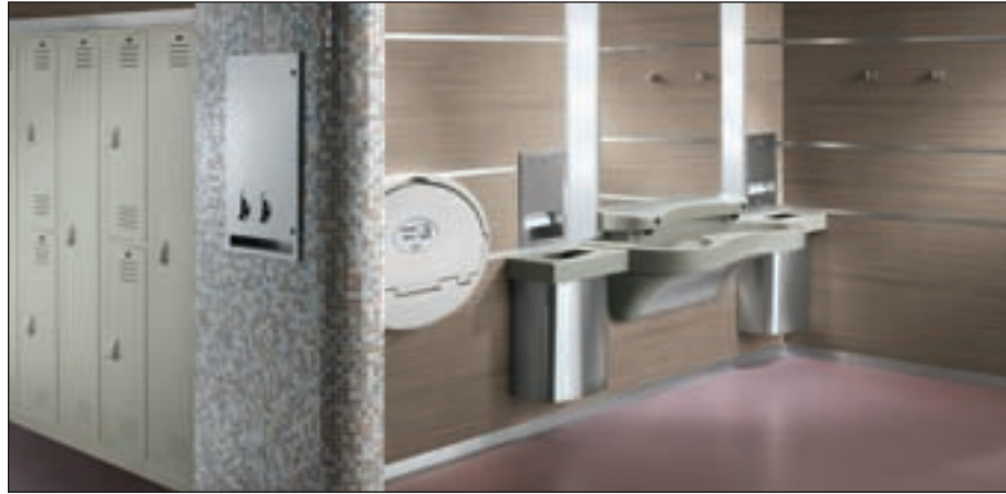
Group handwashing fixtures are a popular choice for green restrooms, since these water-saving fixtures restrict water flow to less than 0.5 gpf. Restroom fixtures, such as partitions and lockers, that incorporate recycled materials make an even greener choice and help earn LEED credits.
