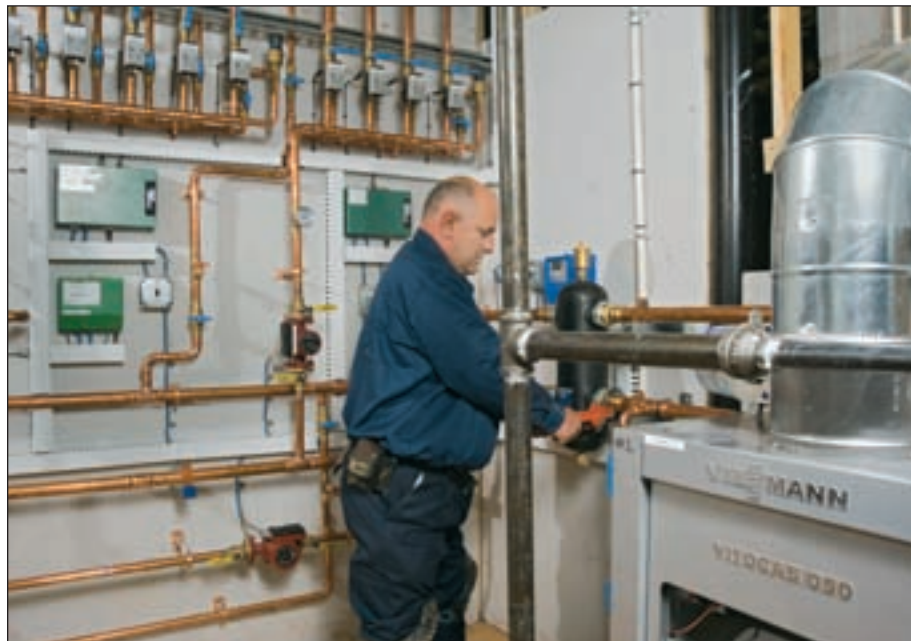
Mechanic Papa Duric completes a connection for the system's Caleffi hydro-separator.
