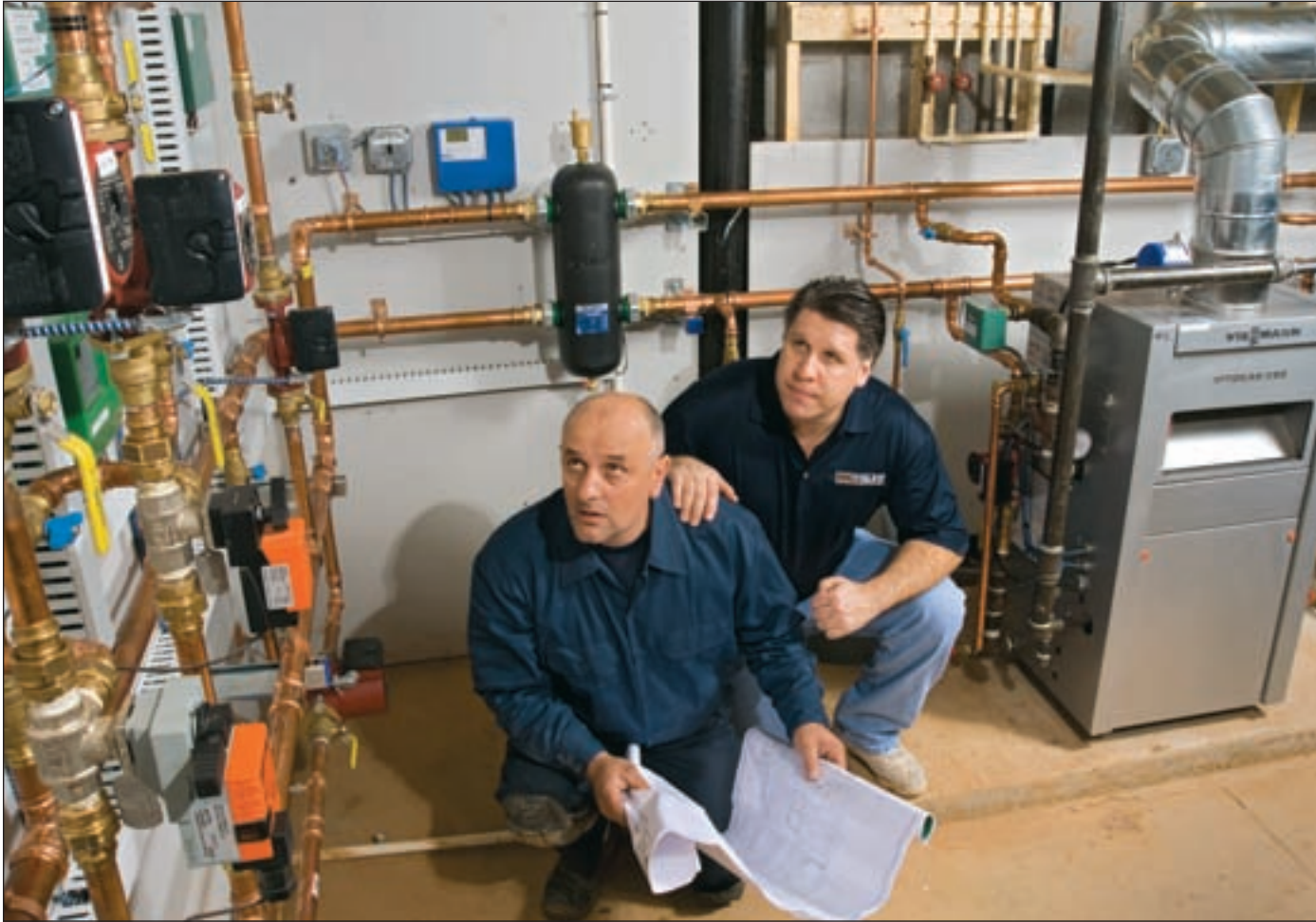
Papa Duric (l), FMI's lead mechanic on the project, and Dan Foley, discuss completion of one of several elaborate mechanical systems at the estate.
