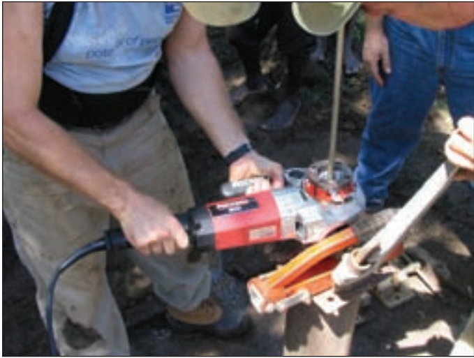
LWI program director Jim Mohney relies on a RIDGID handheld power threader for well repair.
