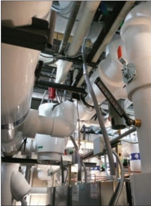
The engine that drives the MAC installation is the TRAK International GeoExchange Ground Source Heat Pump System. The system has four 60-ton heat pumps dedicated to the Source Loop, and two 60-ton heat pumps dedicated to the load loop, providing 145 F hot water.
