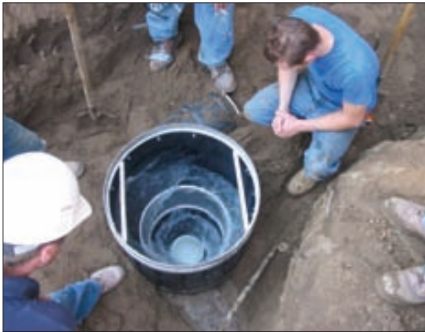
A high capacity vortex filter in action during construction of the Burton School. This pre-tank filter diverts the "first flush" and prevents debris from entering the tank. A single filter can treat roof areas up to 33,000 square feet. (Photo courtesy of Paula Leatherman.)
