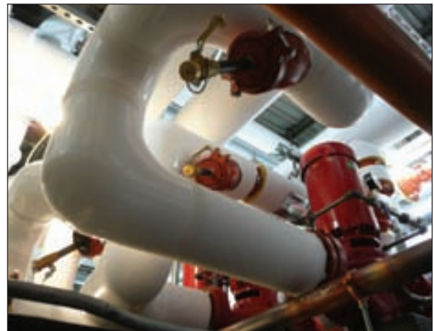
The arena used a dehumidification unit that contained a desiccant wheel that was recharged by heat generated from a 750,000 Btu natural gas hot water boiler. The hot loop piping was extended to this unit in order to use waste heat generated from maintaining the ice to recharge the desiccant wheel.
